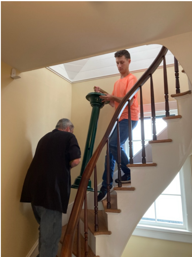
Carrying the replicated 6 th order stand to the lantern room where the current LED optic will be placed on
